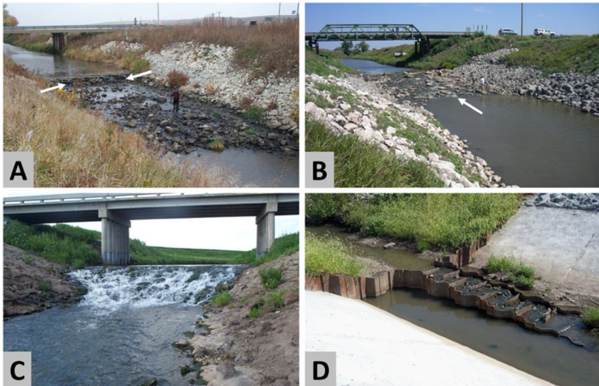
Figure 1. Examples of grade control structures (GCS) in western Iowa streams. Photographs were taken at low-flow conditions. (A) Sheet pile weir with loose riprap slope, originally built at 1:20 (rise : run), but note how rock has moved away from the sheet pile weir (white arrows). (B) Sheet pile weir with 1:20 grouted riprap slope and manufactured blocks intermittently placed in the central low-flow portion of the slope extending above the adjoining rock (white arrow). (C) Sheet pile weir with 1:4 grouted riprap slope. (D) Sheet pile weir with 1:20 fish ladder and steel baffles. This figure is available in colour online at wileyonlinelibrary.com/journal/rra
